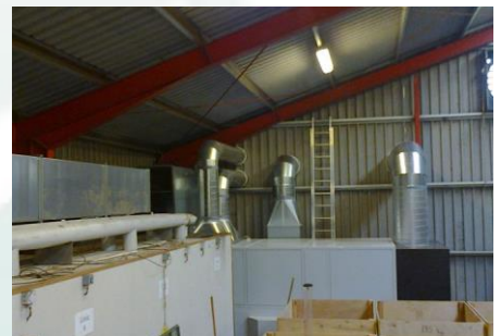
Air duct connected to new adsorption air dryer.
