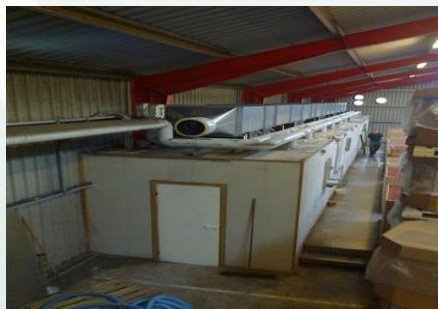
New air duct on plenum to distribute dried air per section.
