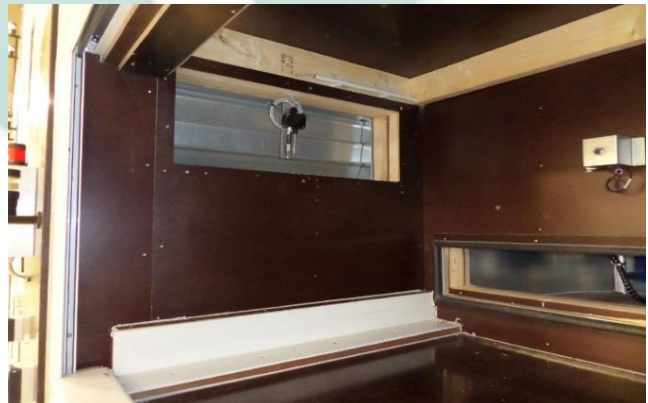
Outlet with T°+HR sensor to control the process.
