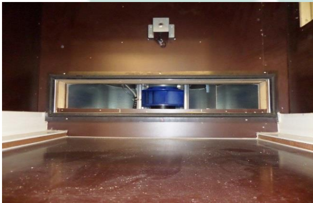
High-pressure fan with flow sensor for each box place.
