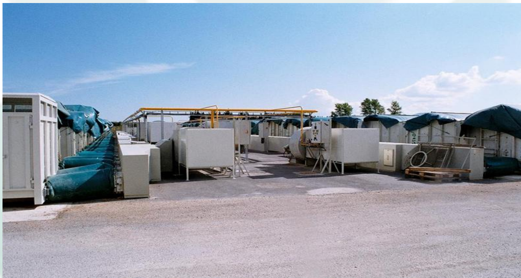
Drying sections with fan, air distribution duct and connections to the containers.
