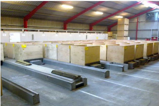
Drying installation before modification; per row boxes a fan
