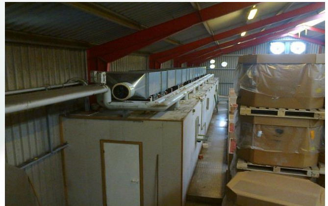
Drying installation after modification; each row boxes individually provided with dehydrated air.
