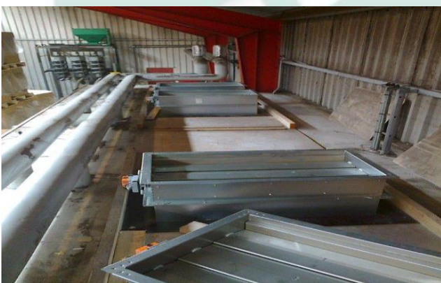
Roof of existing drying installation; installation of valve registers for dry air per row/fan.
