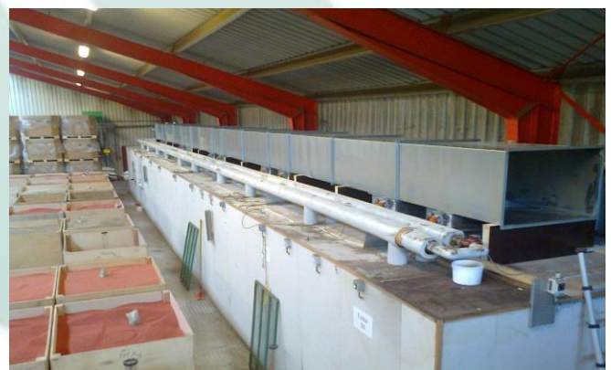
Air distribution duct on top of valve registers. Air from air drier distributed to each drying section.
